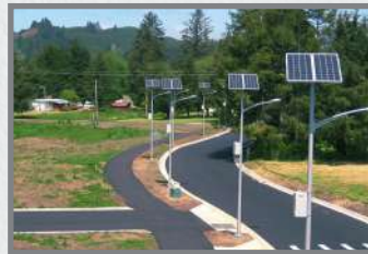
Solar and electric street lights.
