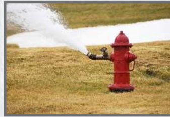
Fire hydrant system
