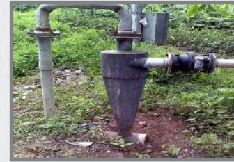
Bore wells for supply of water.
